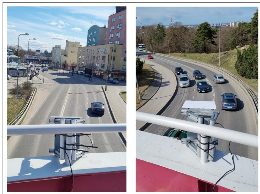
Figure 36. Mounted hardware on both sides of the bridge
